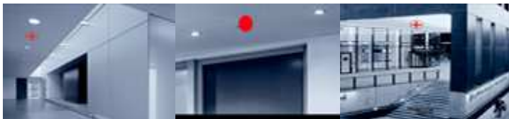
Motion Sensor in Lift landing area, Main Entrances, High Indoor Spaces, Lobby
