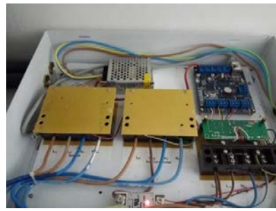
圖一. 安裝在和聲書院全部300個宿生房間的智能電錶。 Fig. 1. The smart meters that were installed in all 300 rooms of LWS hostels.
