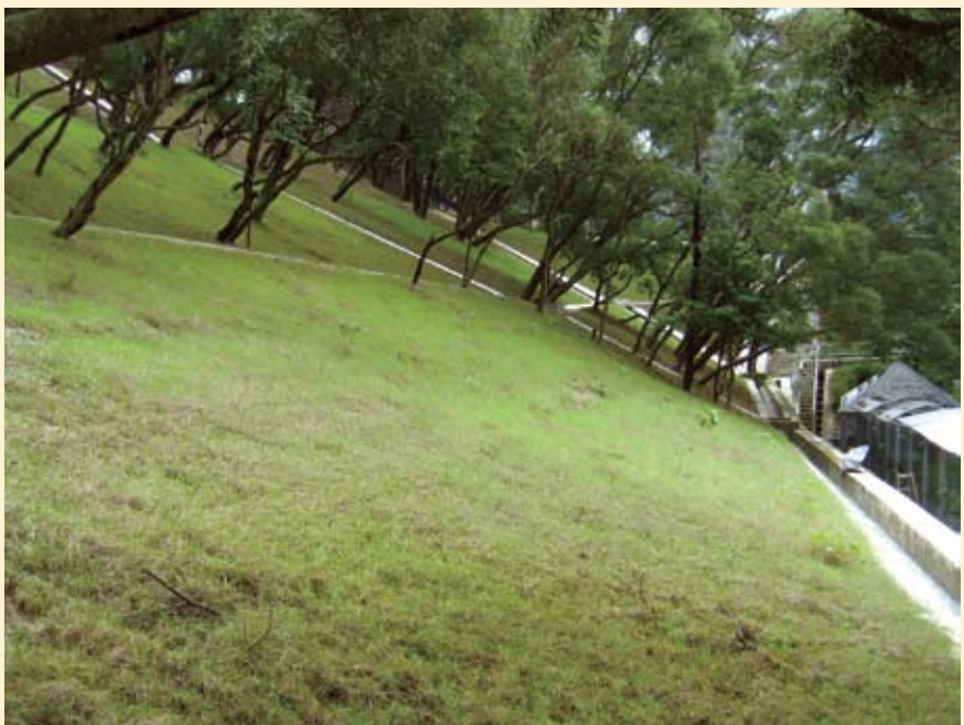
在邵逸夫人樓附近的回填坡，是藉挖坑種植來鞏固的。這種方法可盡量減少移植樹木，部分過程須用人手處理，耗時較長。 A more time-consuming method of stabilization—trench excavation—was used to stabilize this fill-slope near the Lady Shaw Building so tree removal can be minimized. Part of the procedure was carried out manually.
