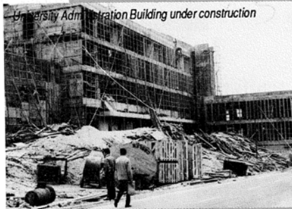
The second building on the central campus – the Institute of Chinese Studies (old wing) near its completion in 1970.
