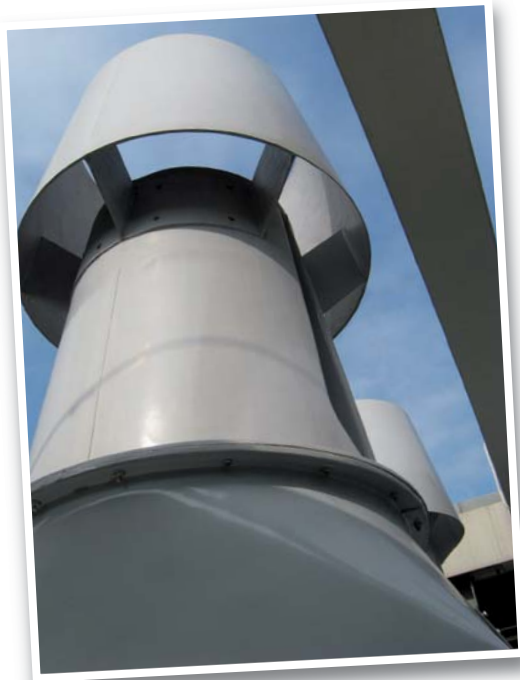
抽風系統設有過濾系統及增強氣流風扇以保護環境 The fume exhaust system equipped with filter systems and booster fans for protection of the environment
