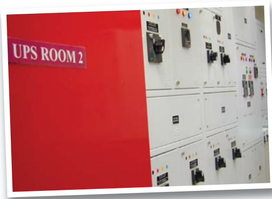
碧秋樓電腦房的不斷電系統從60kVa提升至300kVa Uninterruptible power supply (UPS) was upgraded from 60kVa to 300kVa
