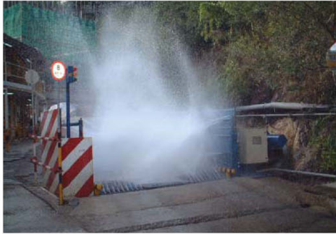
地盤入口洗濯池，可減少附於車輛上的塵土。 A vehicle washing pool at the entrance of a construction site
