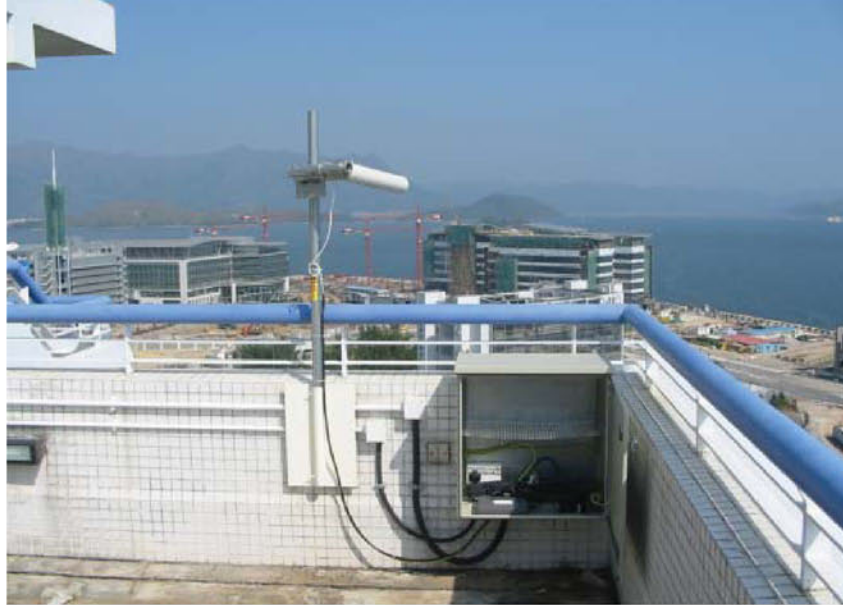
校園東區的無線網絡設施 Wireless network facilities on Eastern campus
