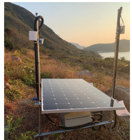
Figure 5. A solar-powered node at Lantau Country Park.
