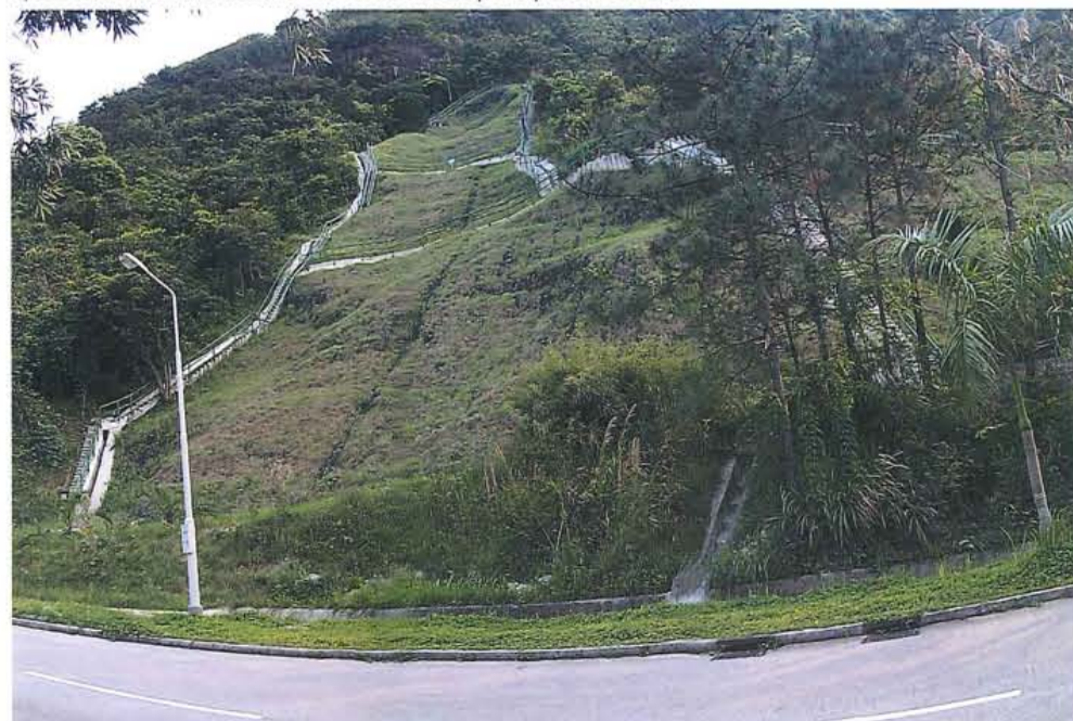
Fig. 2 A steep slope along Campus Circuit Road — once the highest slope on the campus. It has now been made more gentle in addition to being hydro-seeded and covered by an erosion control mat. Over 1,000 soil nails have been inserted into the slope to prevent erosion.
