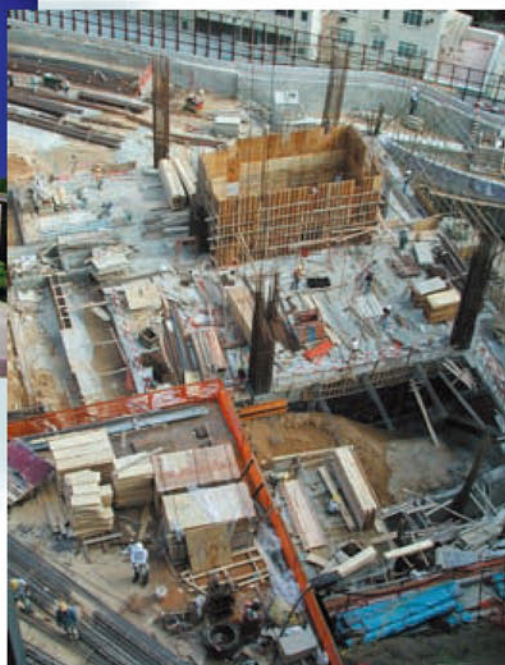
第二期工程學大樓興建工程如火如荼 The Engineering Building Complex Phase II under construction
