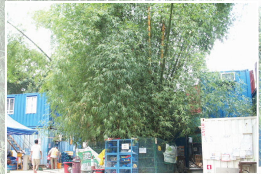
The rare bamboo bush at the construction site of TITB 綜合教學大樓地盤中罕見的竹林
