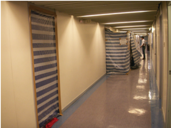
The site with asbestos demolition work is properly sealed according to the occupational safety and environmental requirements.
