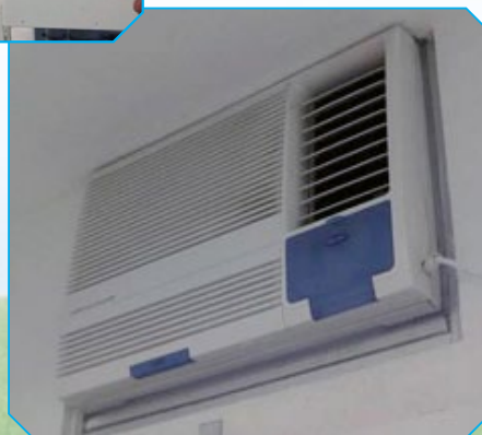
Window-type air conditioner with energy efficiency label 1 for student bedroom
