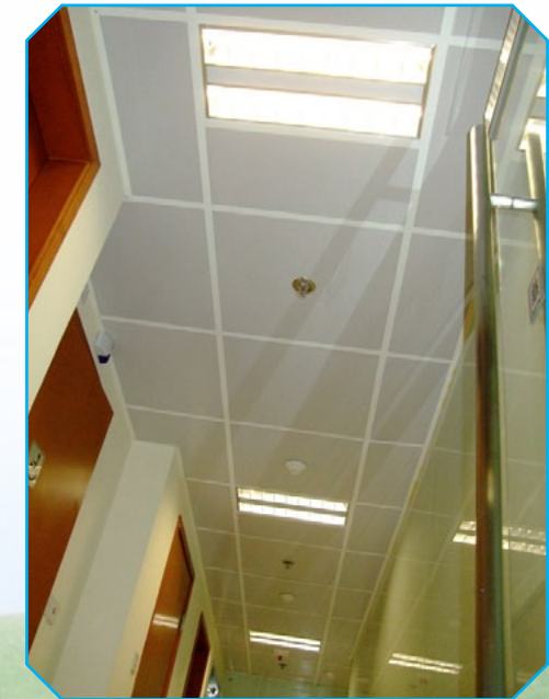
LED lamps replace tungsten halogen lamps in selected offices and lecture theatres
