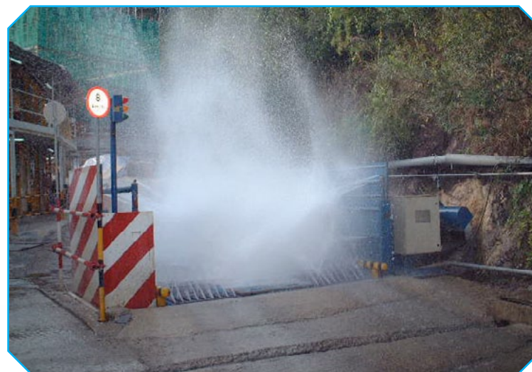
Wheel wash is installed at the entrance of construction site to reduce dust emission
