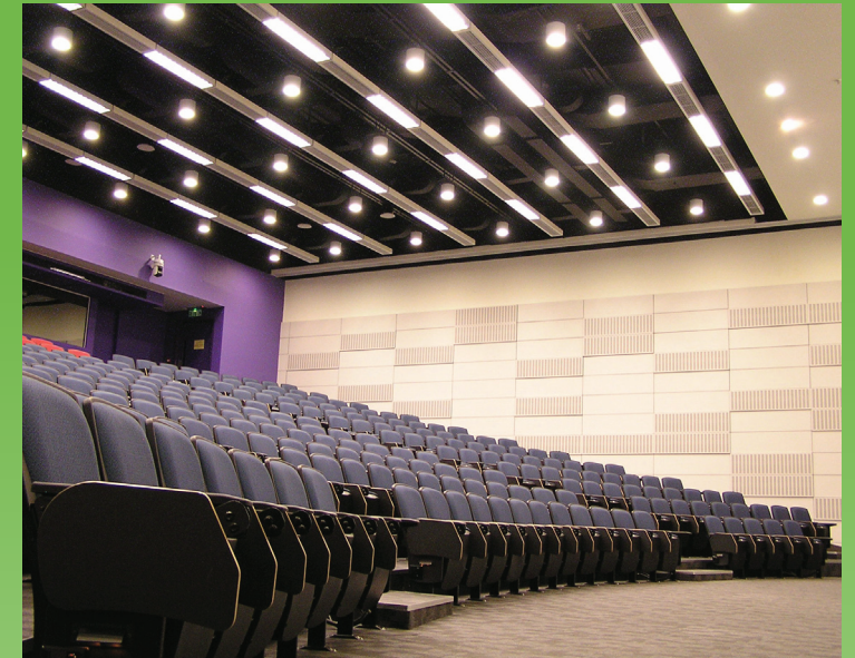
Variable air flow and energy-efficient light fittings in lecture theatres
