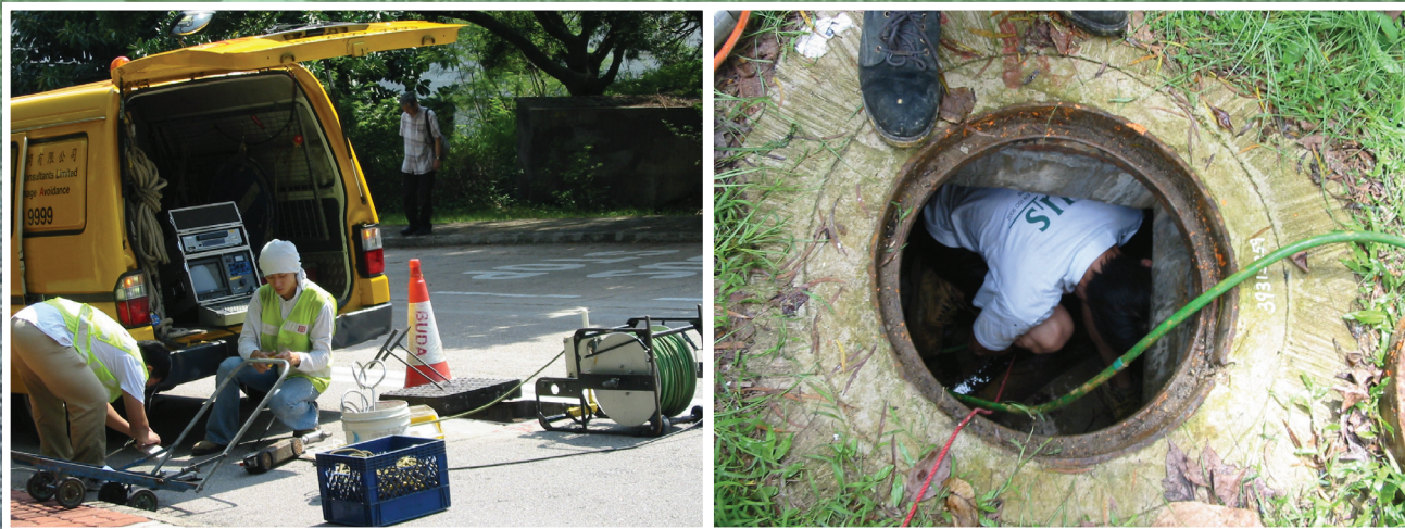
Testing leakage of underground facilities by consultants 顧問人員測試地下設施是否有滲漏
