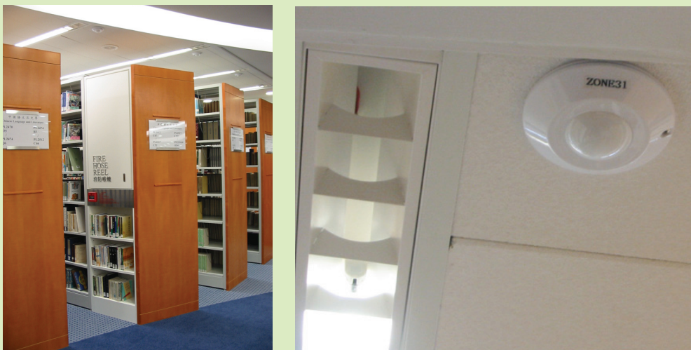
Occupancy sensors are installed to control lighting in the library
