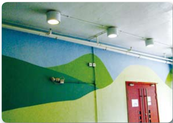
Occupancy sensors are installed to control the lighting of corridors. 走廊安裝了自動感應器控制照明系統。
