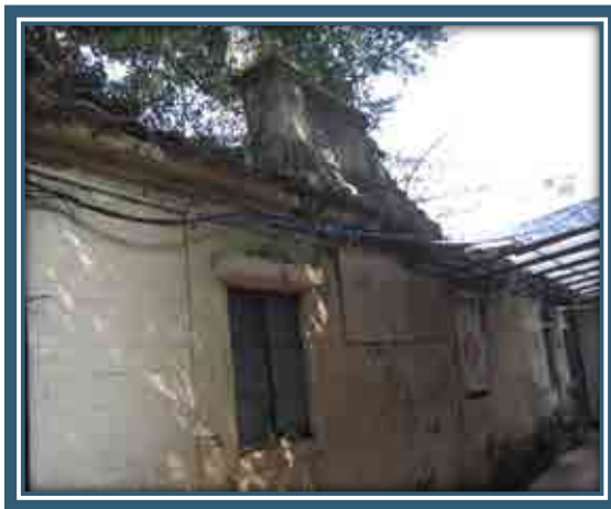
Photo: The façade still bears the Chinese characters of “Catholic Church” (partially collapsed) in the above and an old plaque that reads “Shung Tak School.”
