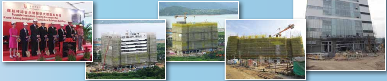
From start to finish – different stages of constructing the Lo Kwee-Seong Integrated Biomedical Sciences Building 由奠基興建到竣工的羅桂祥綜合生物醫學大樓
