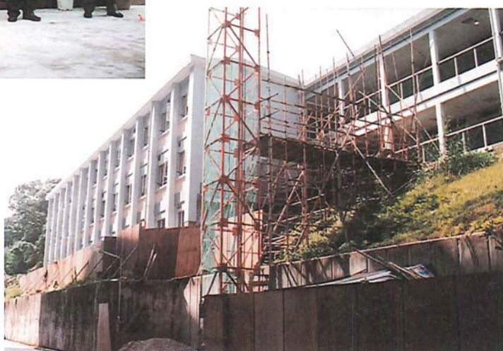
崇基教學樓群第七和第八座翻新工程 Renovation of building blocks VII and VIII on Chung Chi campus
