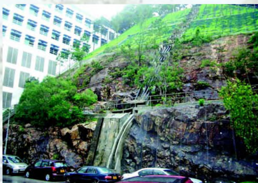
📍 Beside the Mong Man Wai Building Top half of the slope — on the left, fiber soil is used while, on the right, ordinary spray grass technique. The former is ideal for short growth time span and the latter is better for a longer time span.
