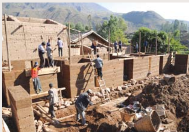
Local villagers have been fully engaged in the construction of the first village house prototype.
