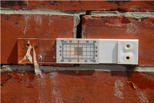
Ex: mechanical strain gauge used to measure the growth of a crack in a masonry foundation.
